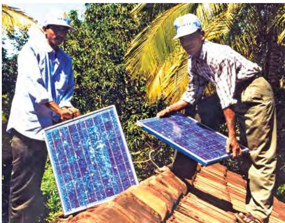
SOLAR HOME LIGHTING SYSTEM Designer/Manufacturer: SELCO-India © SELCO-India
